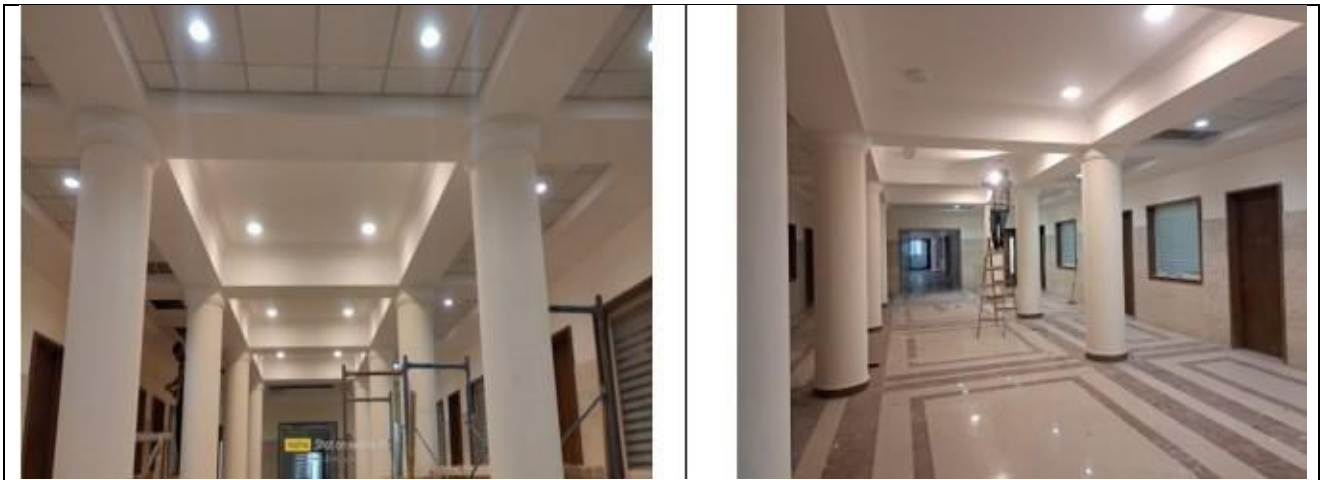
Energy Efficient Appliances Usage: Use of LED lighting and lamps (New Abbes Campus, Alexandria University)
