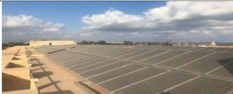
Solar photovoltaic with a capacity of 220 kilowatts on the 2000 m 2 roof top of the building of the Mechanical Engineering Department at the Faculty of Engineering
