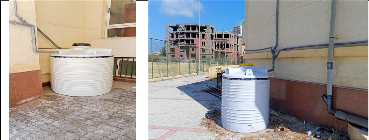
Air conditioning water collection and reuse unit - Faculty of Engineering
