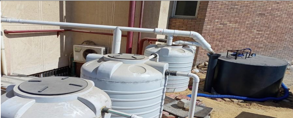
Wastewater treatment unit at Faculty of Engineering
