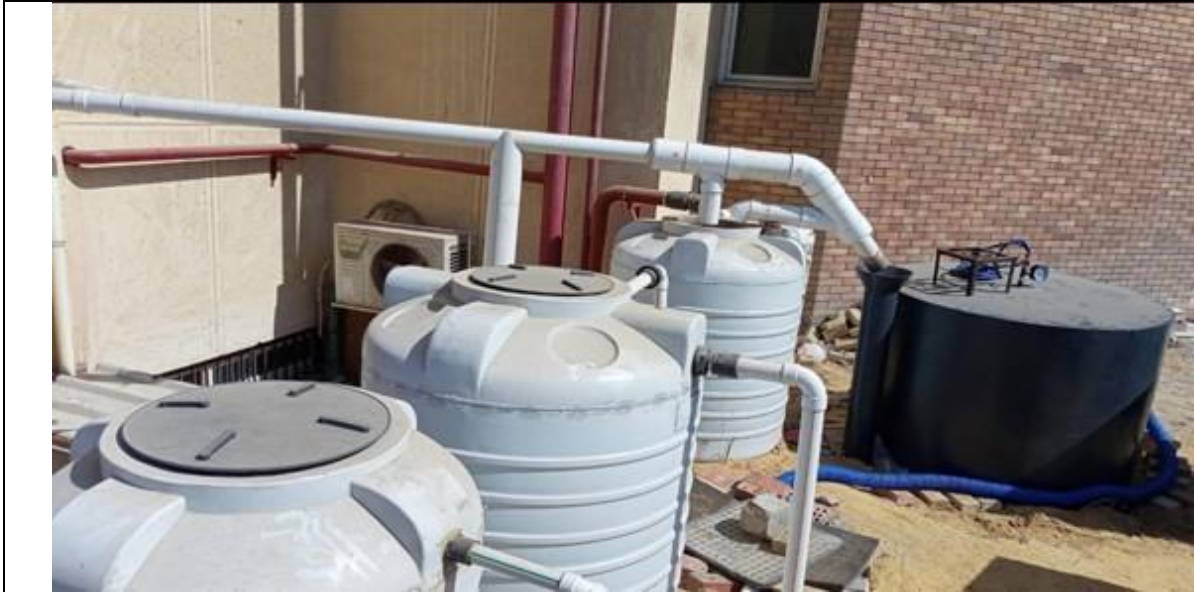
Wastewater treatment unit at Faculty of Engineering
