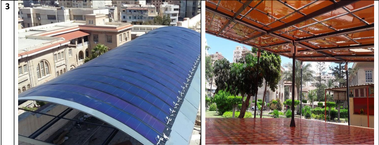
3 BIPV Roof Pergola, Faculty of Science in Moharram Bek (Alexandria University)
