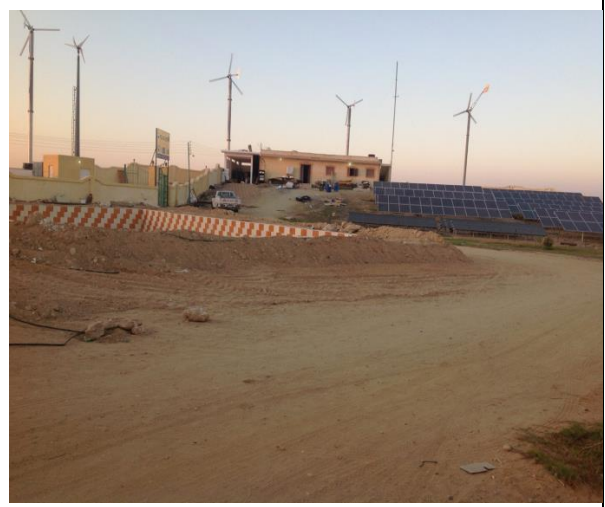
100 KW Hybrid Wind/PV System (50 KW PV and 50 KW Wind)
