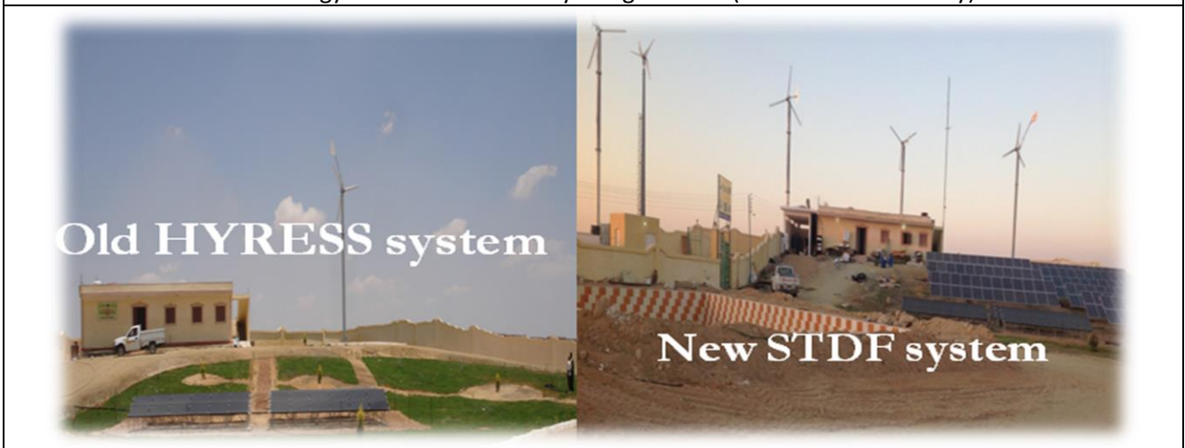
Example of Windmill and Solar Panels (Solar Energy Center at the Faculty of Agriculture - Alexandria University)
